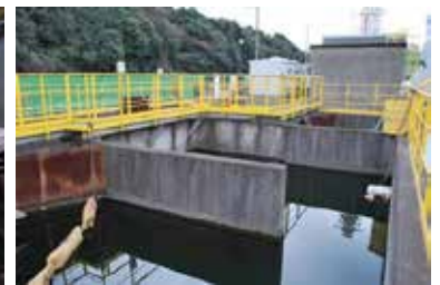
Oil-water separation tank is installed
